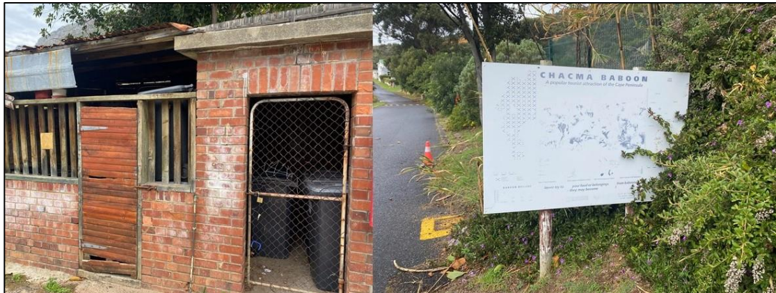
Figure 9. Baboon damage to bin room and faded signage at Miller's Point Resort.
