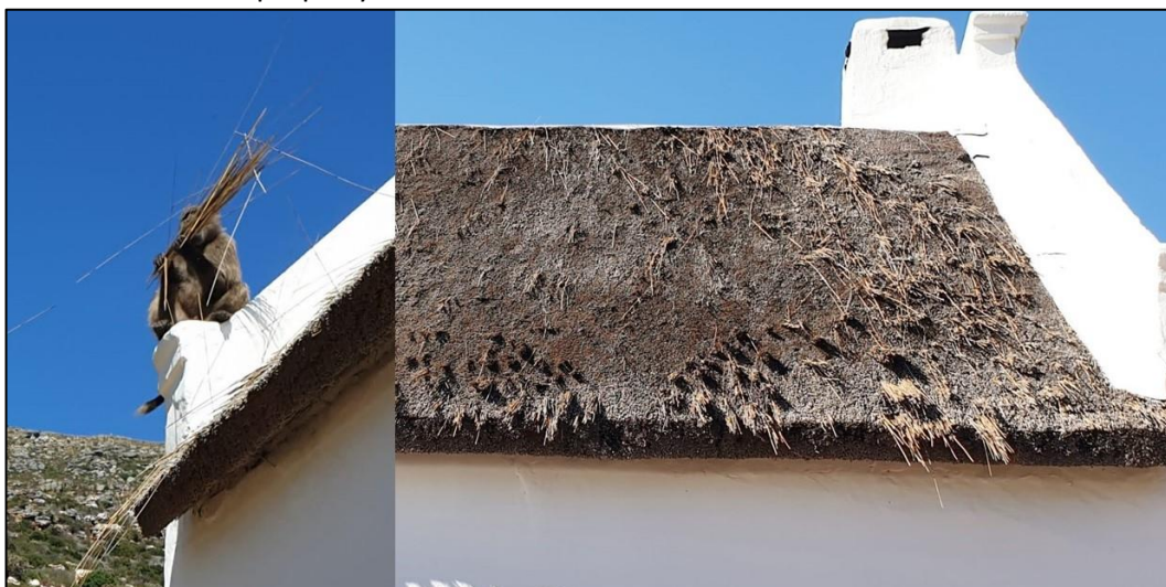
Figure 2. Baboon damage to a thatched roof. Mitigation measures were discussed with the resident.
