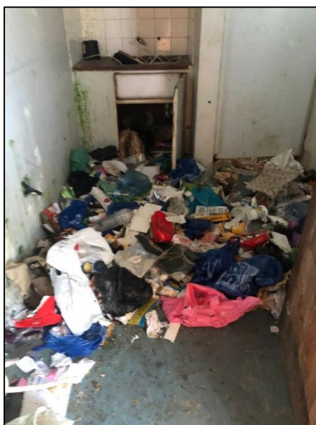
Figure 10. Improperly secured waste room at the ladies' flats at Waterfall Barracks.
